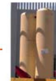
Heat Storage Tanks
