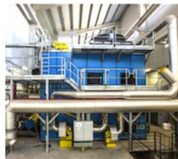
POLYTECHNIK Biomass Energy Biomass Boiler Plant 4,810 kW
