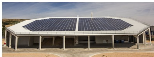
Solar Power / Photovoltaic
